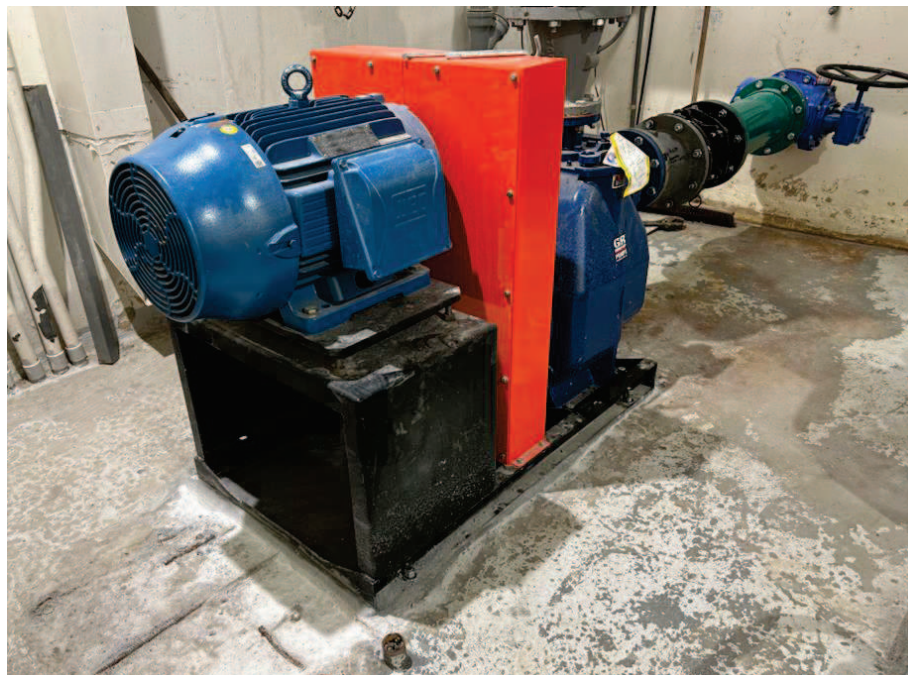
Photo 1 – New 50 HP Sewage Pump
