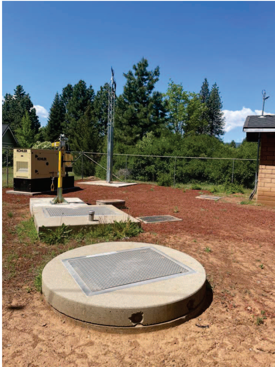
Photo 2 – Bartel Lift Station Antenna, Emergency Generator, and Davit Crane
